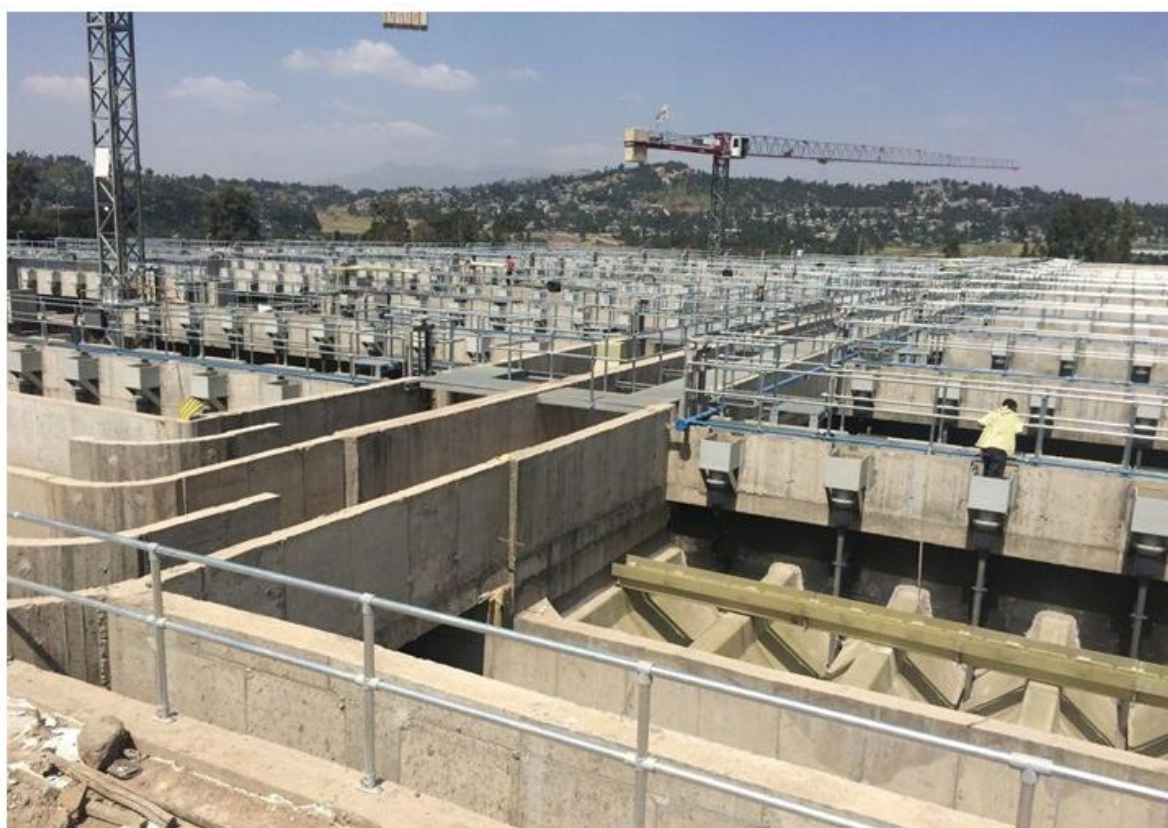
Figure 102 Akaki Kality UASB Wastewater treatment plant, Addis Ababa
